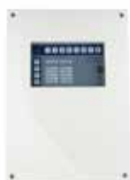
Fire Alarm Panel
